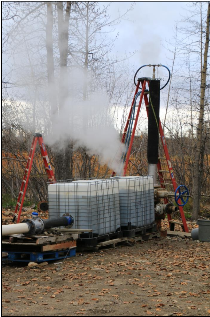
Figure 1. Surface equipment utilized for airlift of PS 13-1. The magmeter is in the silver spool between the black and white parts of the flow line. The black heavy large diameter hose serving as a standpipe on the top of the wellhead was needed to prevent water from flowing out the top of the wellhead. The clamp holding the aluminum tubing is visible on top of the standpipe. The blue hoses are the air lines coming from the trailer mounted air compressor.
