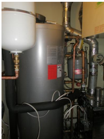
Viessmann 2: Utility Room
