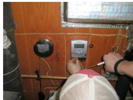
Wiring the DL2 data logger and the Control Unit
