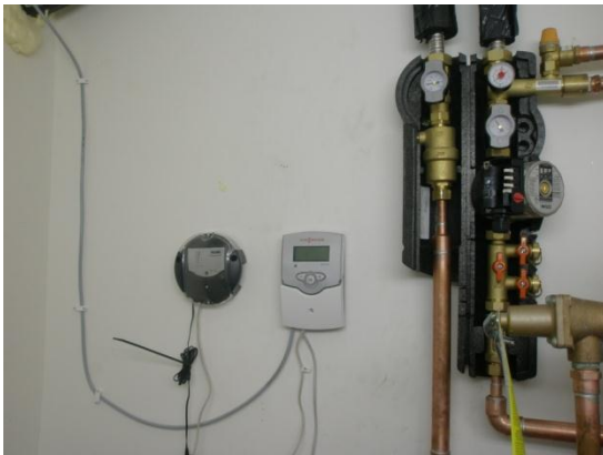
Viessmann 1: Utility Room
