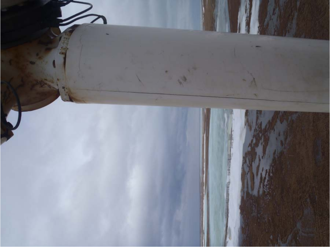
Picture 2: Blade Crack and Corrosion
