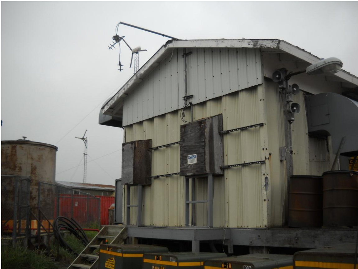
Picture 1: Damaged communication antennae mast
