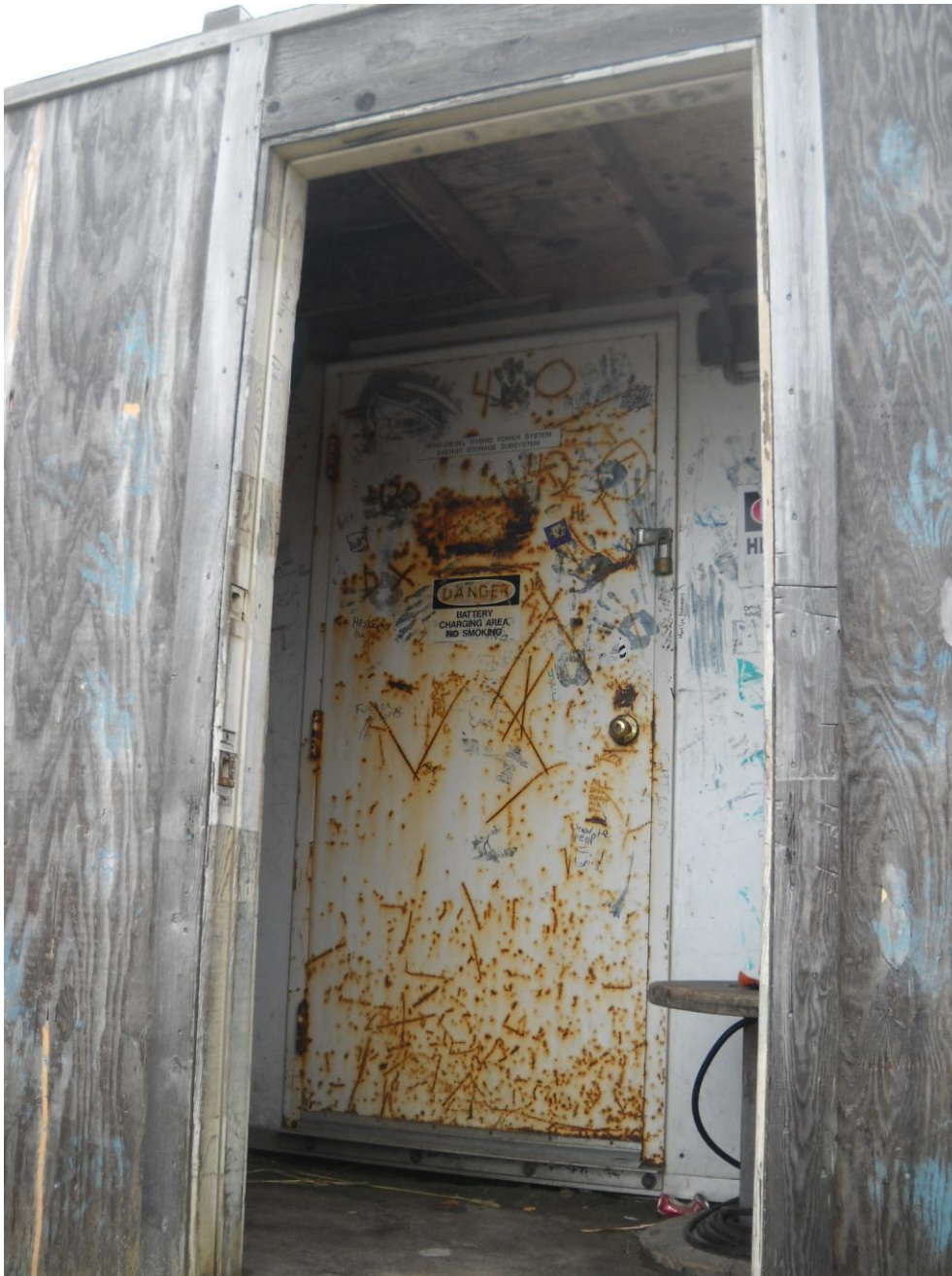
Picture 3: Corrosion and vandalism to ESS entrance.
