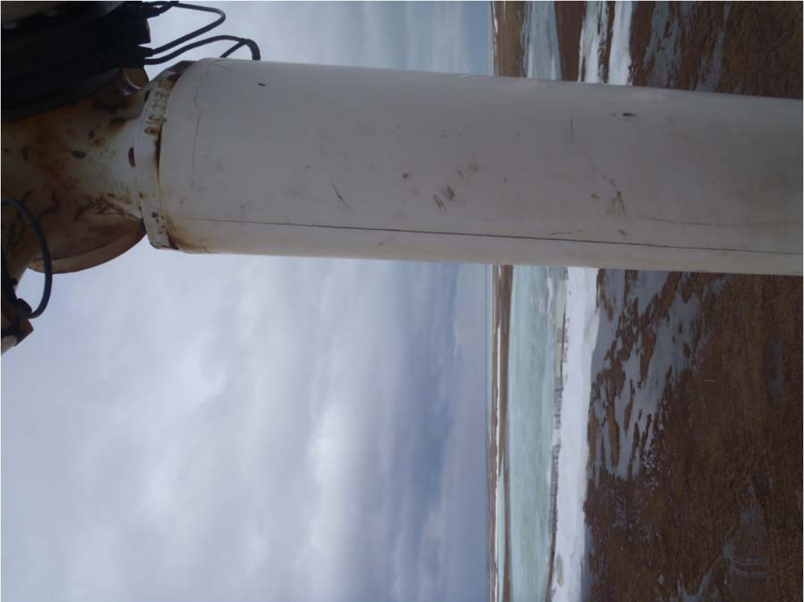
Picture 2: Blade Crack and Corrosion
