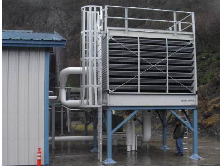
Figure 3: BAC Cooling Tower Used by CEC
