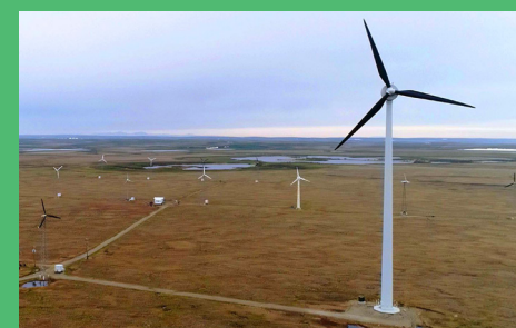
One of two 900-kilowatt wind turbines tower over the almost 3-megawatt Kotzebue wind farm. The farm is a focus of a proposed renewal of the Converter-Dominated Power Systems award.
