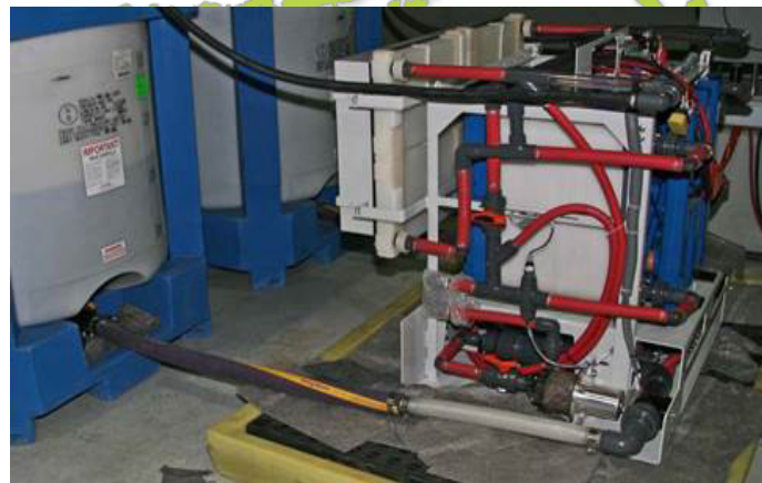
5kW Flow Battery storage system from Prudent Energy. Photo Credit Julie Estey, ACEP.
