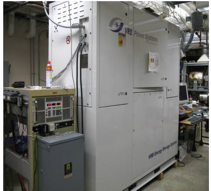
Original first-generation 10kW VRB Battery system tested at the University of Alaska. Photo Credit ACEP.
